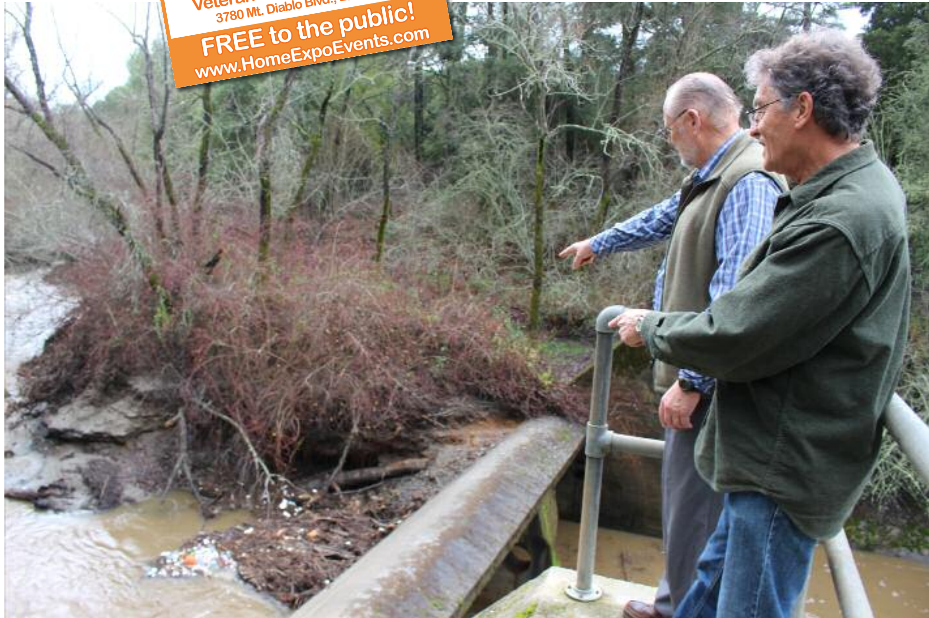
Brian Waters, foreground, and Reginald Barrett of Friends of Orinda Creeks look at debris at what is known as SP201, an East Bay Municipal Utility District "drop structure," or dam, that gets clogged and has prevented native rainbow trout from migrating upstream. Photo Chris Lavin
